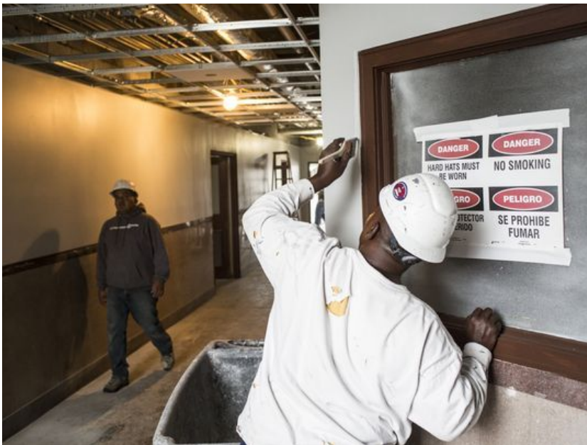
Workers are busy inside the Universal Life Insurance building March 16, 2018. Owners and architects Juan Self and Jimmie Tucker are closing in on completion of a $6.2 million renovation intended to create a showcase of history and sustainability and a collection of resources dedicated to growing disadvantaged businesses. Self+Tucker Architects and the City of Memphis Business Development Center are expected to move into 480 Dr. Martin Luther King Blvd. this spring. (Photo: Brad Vest / The Commercial Appeal)
