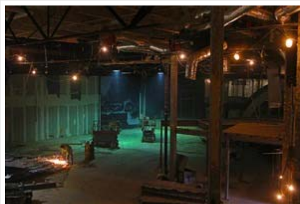
Flintco Constructive Solutions is the general contractor for the renovation of the 44,500-square-foot Lorraine Motel building at the National Civil Rights Museum.
